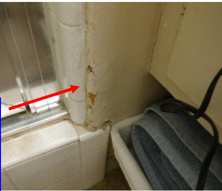
...the wall adjacent to the master shower shows water damage...
