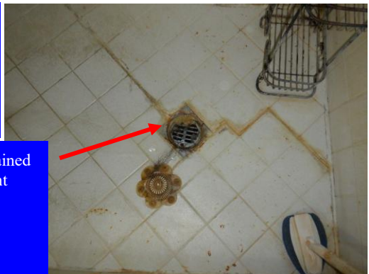
#304: The S-bedroom W-window sill is water damaged...
