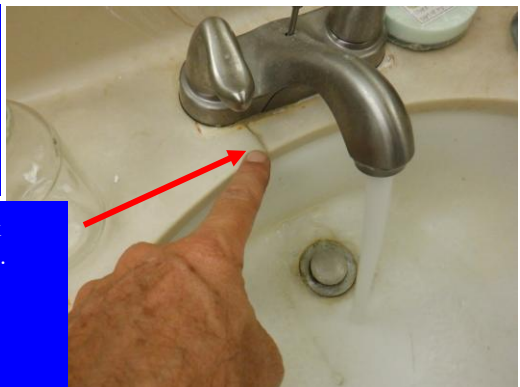
...as well as water damage just outside the shower..
