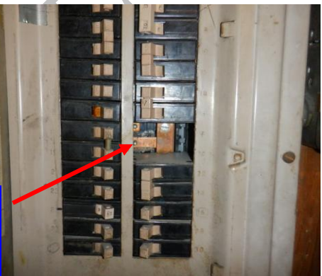
The NW-electrical distribution panel has an unused breaker opening...
