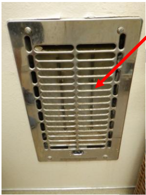
#114: The wall mounted coil heaters noted here and at other units must be removed...
