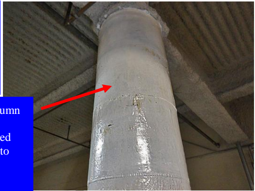
A support column at the pool equipment area required re-supporting the base due to excessive corrosion of the embedded steel reinforcing bars
