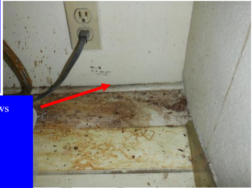
...the hall bath shower panel is detaching from the wall...
