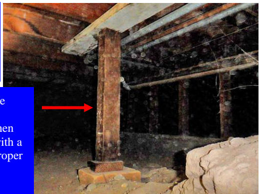
The fireplace hearth extension form boards were not removed
