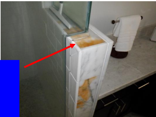
...and the loose rear wall blocks can be pushed causing powdered mortar to fall from the joints
