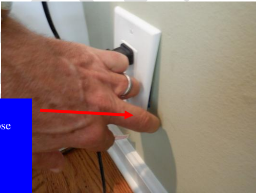
...which is prohibited as it also lacks a vent where the alternate configuration see here is an improvement
