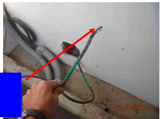
"Buzzing" noted at the left 200 amp breaker
