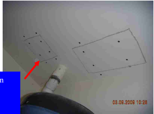
Weep screed needs additional soil clearance
