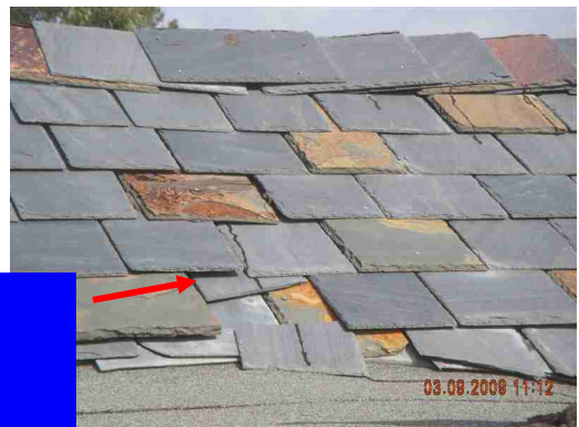
Missing slate roof tiles/exposed nails
