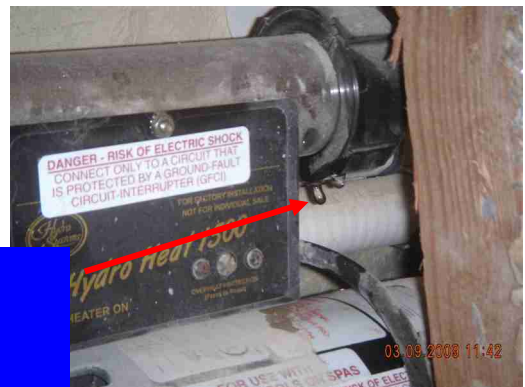
Tankless water heater vent discharging below combustible deck framing
