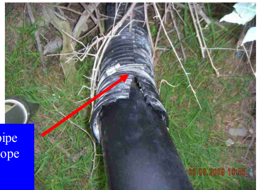
Waste pipe secured with tie-down strap
