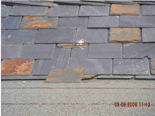
Missing slate roof tiles/exposed nails
