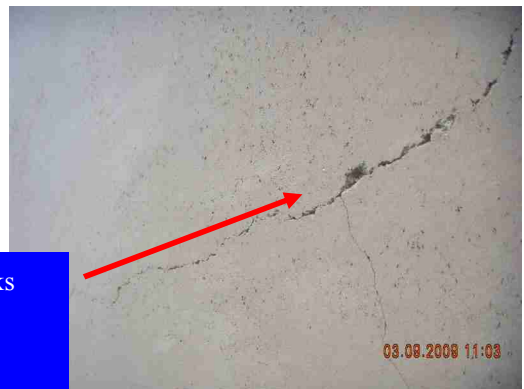
Deterioration of the S side-yard stairway stringer (close-up below tread)
